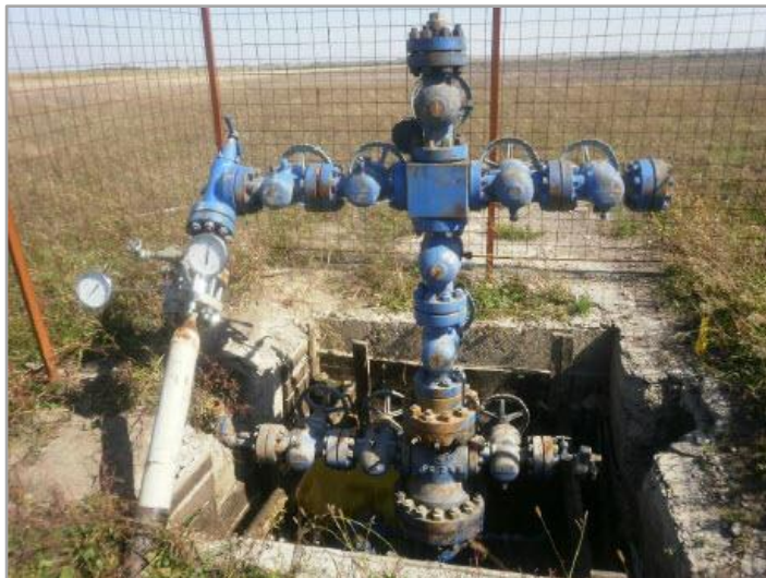
Figure 2 - Cimauti-1 Well Head (Suceava)
